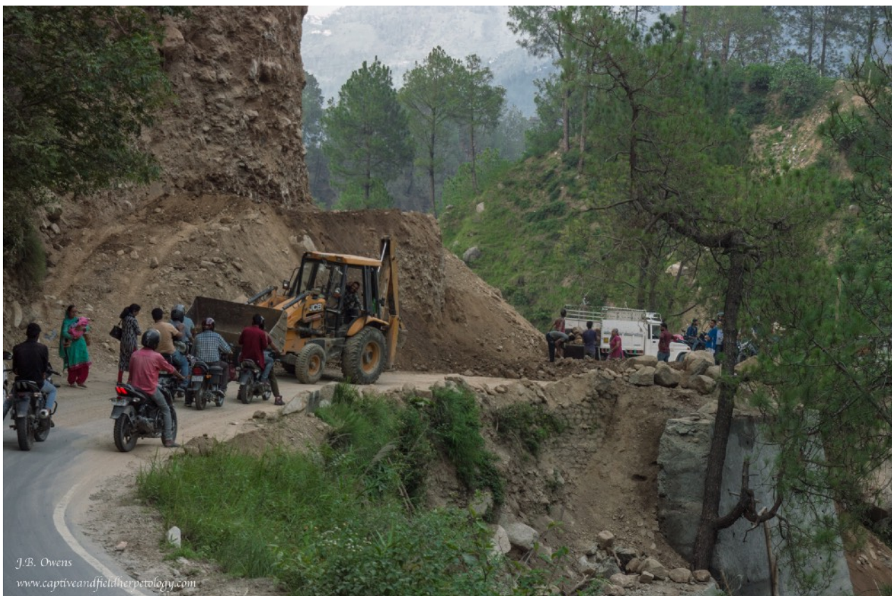
Figure 8. Workers beginning to clear one of many landslides on the drive to Chamba. Caused by frequent rains and steep cliffs.
